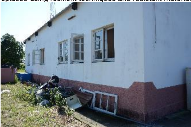
Chinamacondo Health Clinic to be rehabilitated, in September 2021. Damaged windows and roofing will be replaced using resilient techniques and resistant materials.
