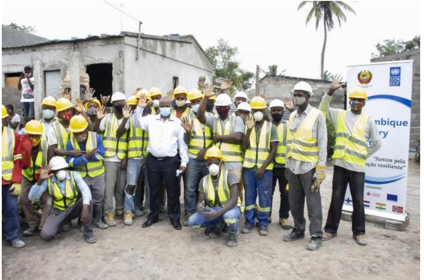
Local masons working on the UNDP Recovery Facility housing rehabilitation project in the city of Beira, Mozambique on 07 December 2020. 320 houses damaged by the cyclone in Beira are being restored using resilient construction techniques. Photo by UNDP.
