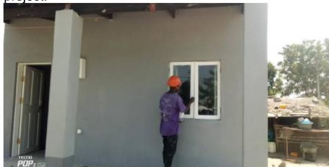
On-going housing construction in Mandruzi resettlement neighborhood, in September 2021. 160 houses are in the project.
