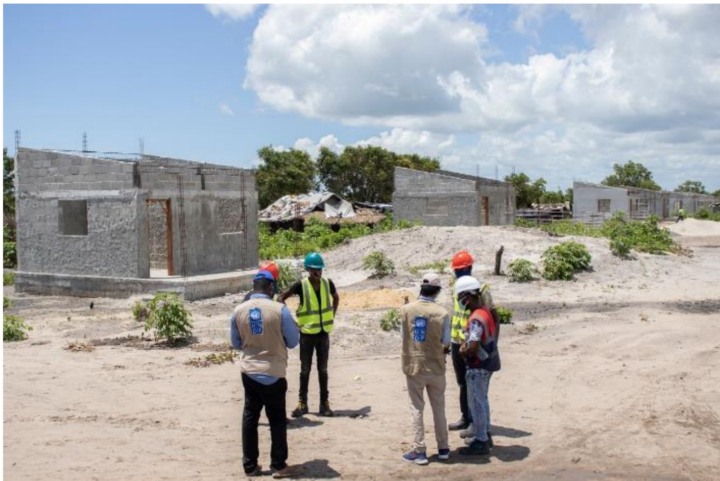
Single-family resilient houses under construction with a roof-covered area of 34 m 2 each. This is a 'evolutionary housing model' where households can expand the structure or develop new functions for the rooms in the future, according their needs and preferences. Photo by UNDP.
