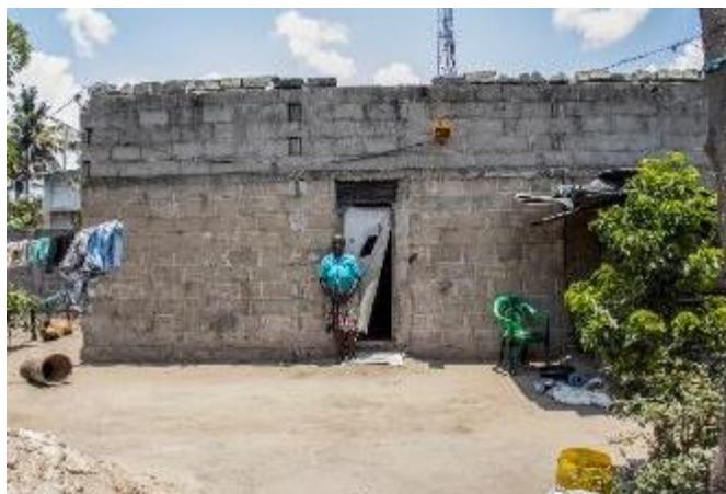
Ms. Nhawa Domingos's house before rehabilitation, in November 2020, in the peri-urban area of Beira city where hardly affected population live.
