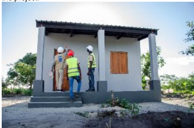
On-going housing construction in Mutua resettlement neighborhood, Dondo, in August 2021. 200 houses are in the project.
